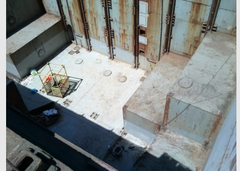
The Crawler is able to inspect even hard-to-reach regions like cargo holds.
